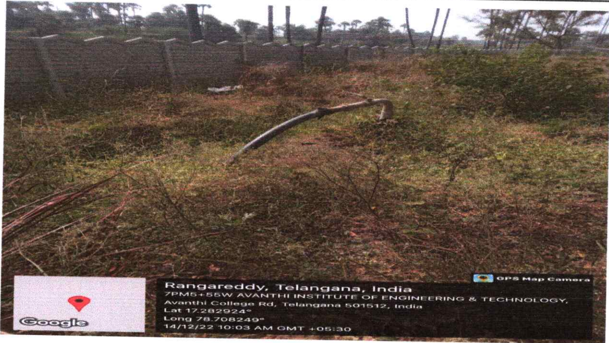
7HP Motor capacity was installed near the Near Main Block
