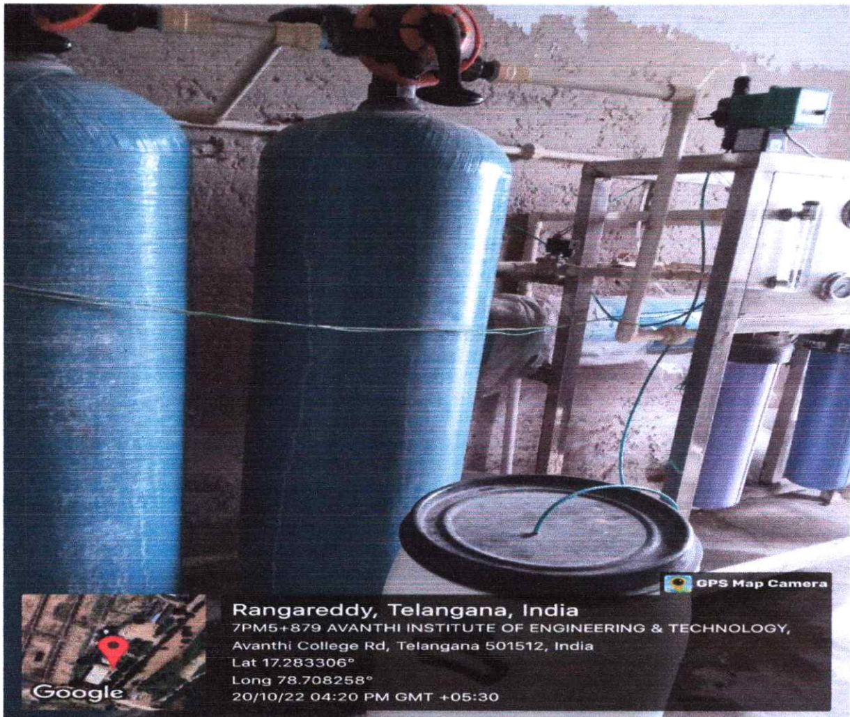
RO plant purified water Plant
